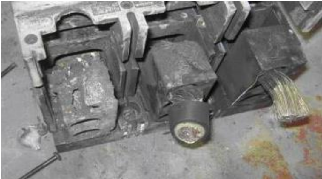
Damage to circuit breaker feeding a capacitor bank. A thermal examination would have detected abnormal heating
